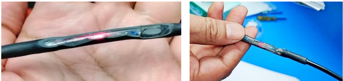
Figure 22. Twisted connection points between the fiber optic cable showing damage with red crack points visible.
