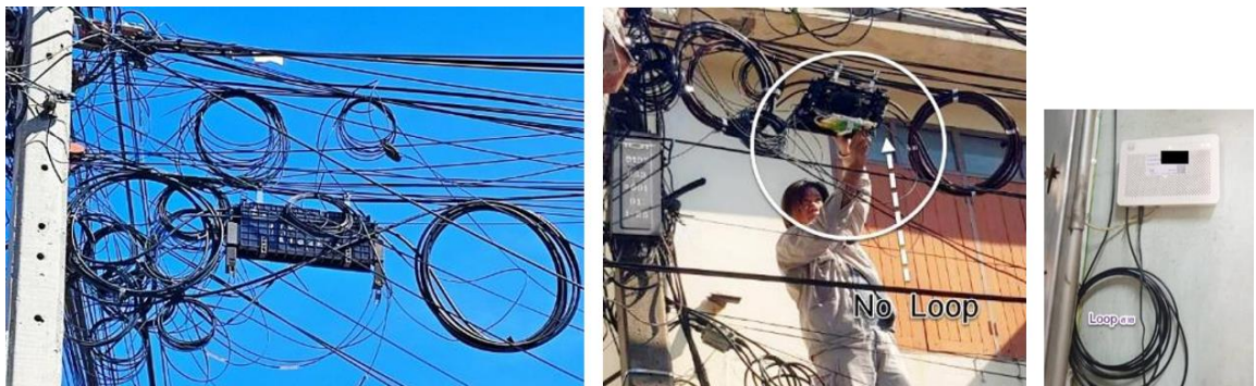
Figure 12. Optic Drop Wire Position at SDP Cabinet, No Looping Allowed (Middle Image)
