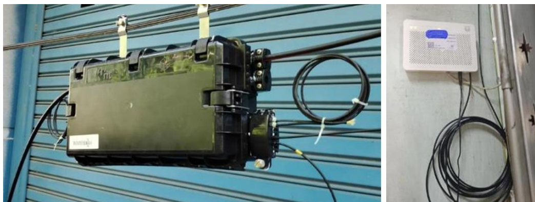
Figure 1. OFTK cables connected at the SDP/ODP cabinet and ONU equipment
